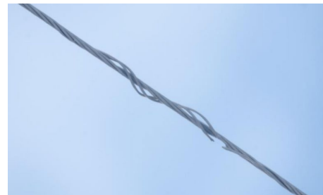
Image: Example of a broken conductor strands that can be identified through early FortisAlberta's early fault detection technology.
