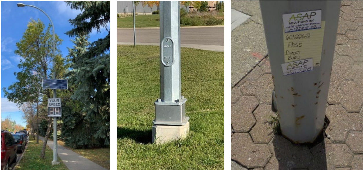
Figure 6 – Existing attachments (left), breakaway poles (center), direct buried (right)
