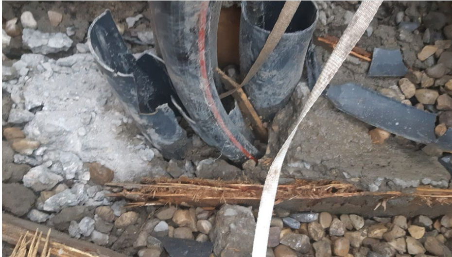
Figure C3.1 Ducting damaged while pulling cable.
