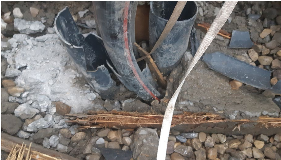
Figure C3.1 Ducting damaged while pulling cable.
