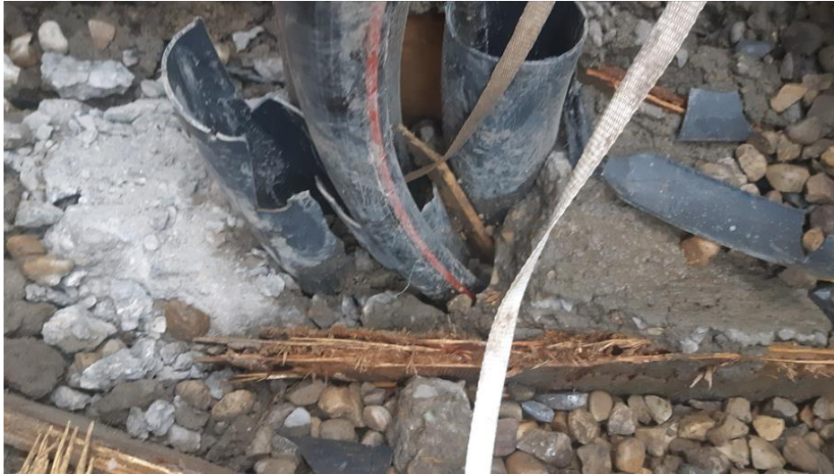
Figure C3.1 Ducting damaged while pulling cable.
